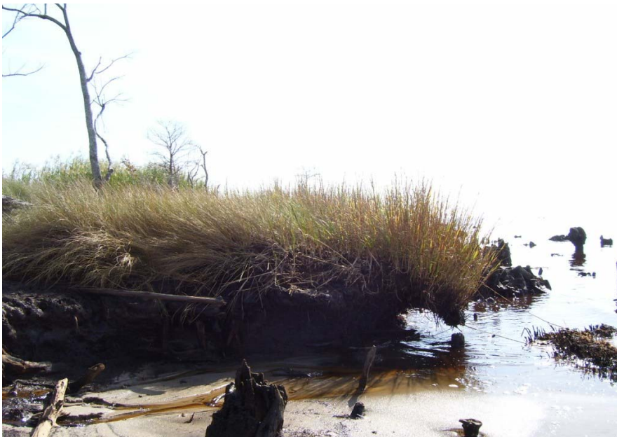
Figure 2.6 Fringe wetland undermining at project shoreline (Author's Photo)
