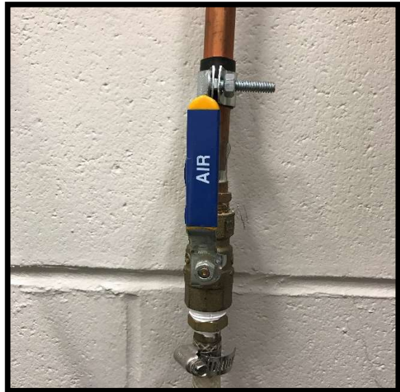
Figure 2b: Air Valve Open
