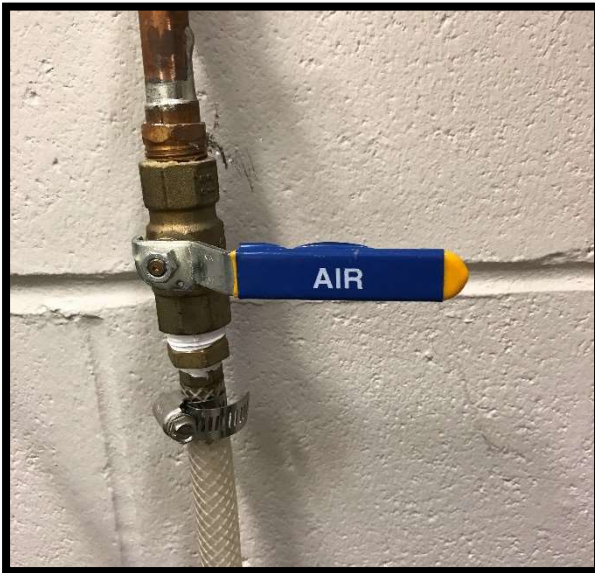
Figure 2a: Air Valve Closed
