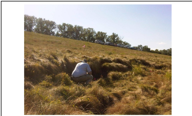
Fig. 1. Typical levee slough (or slump) slide. This one appeared during the major flood event in the Spring of 2011
